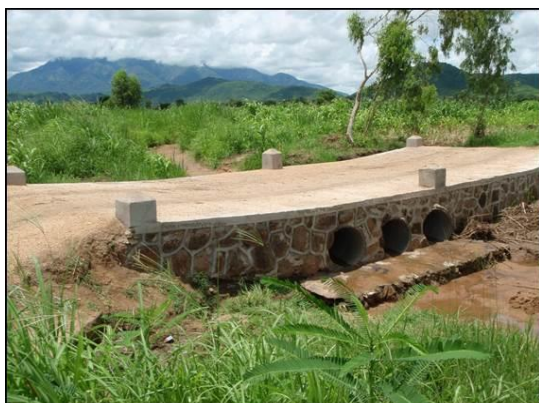
Bridge to site – employed local village workers to assist in construction of bridge
